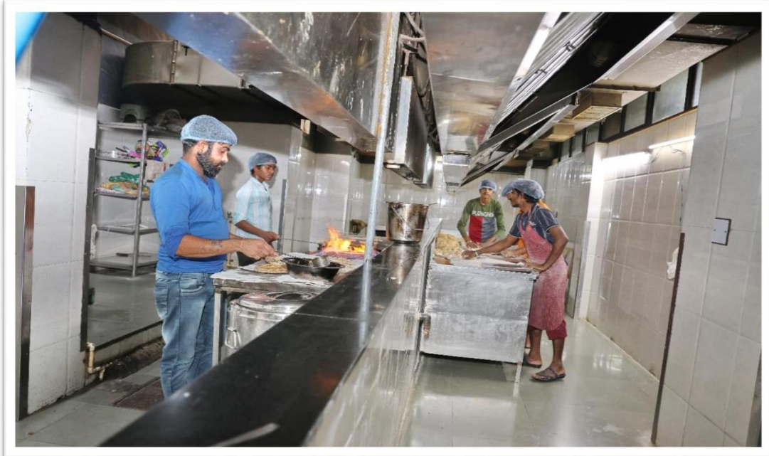
'Aswad' Mess –Kitchen with AHU
