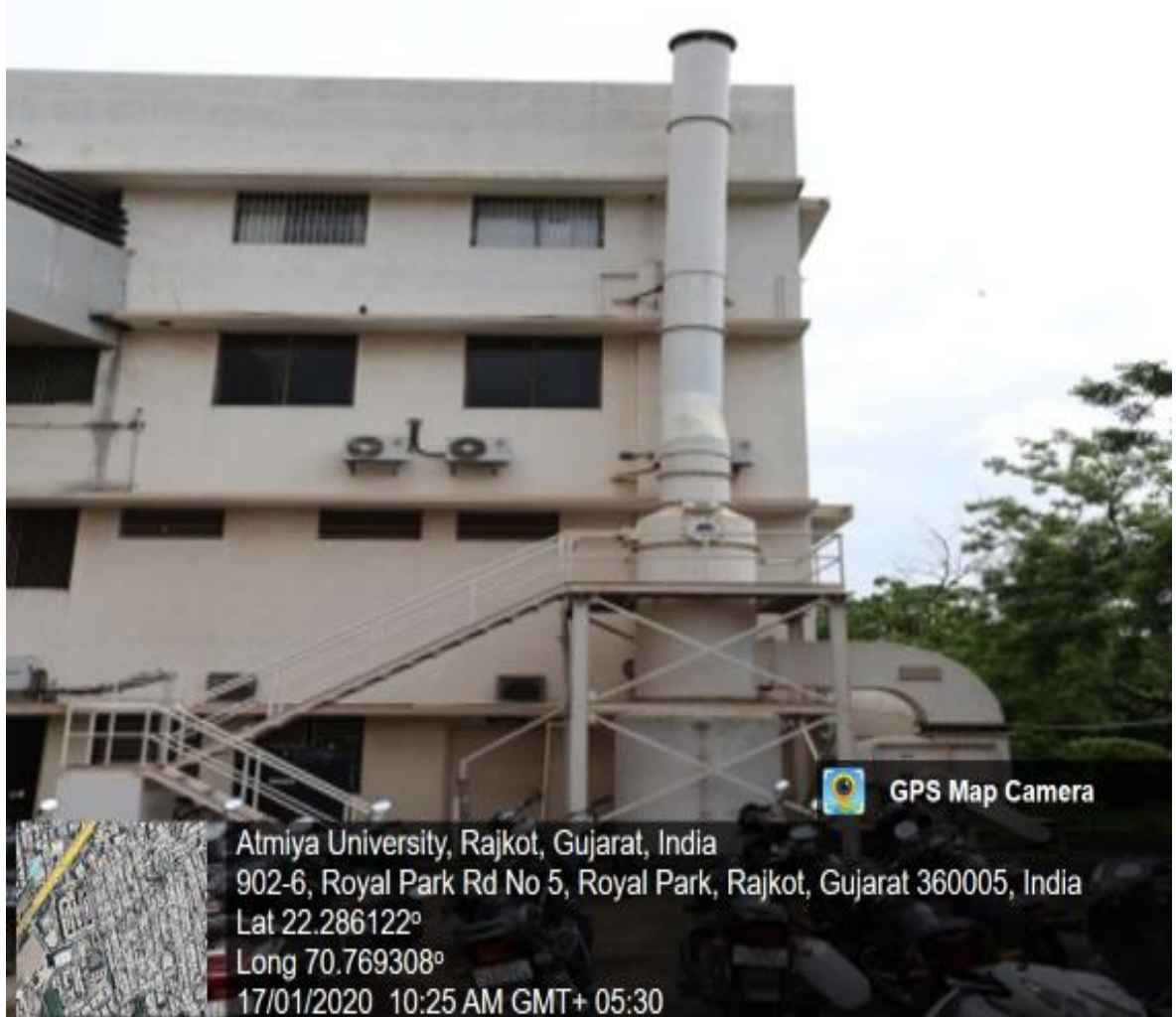
Wet Gas Scrubber
