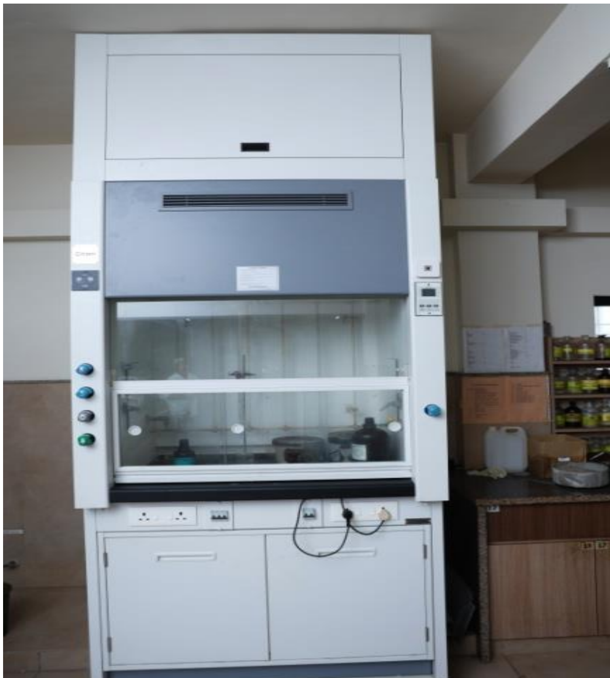
Fumehood at Chemistry Laboratory
