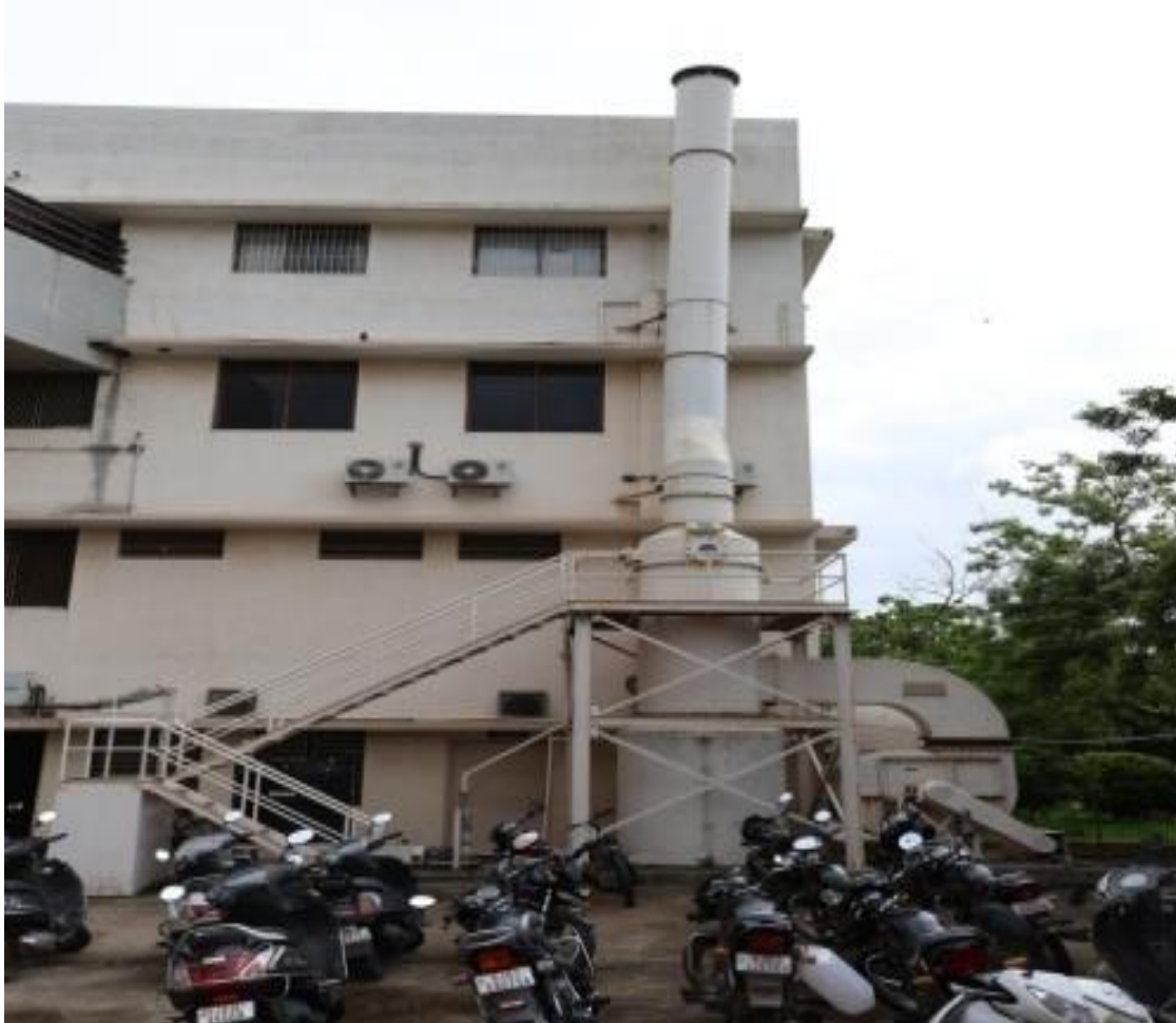
Wet Gas Scrubber
