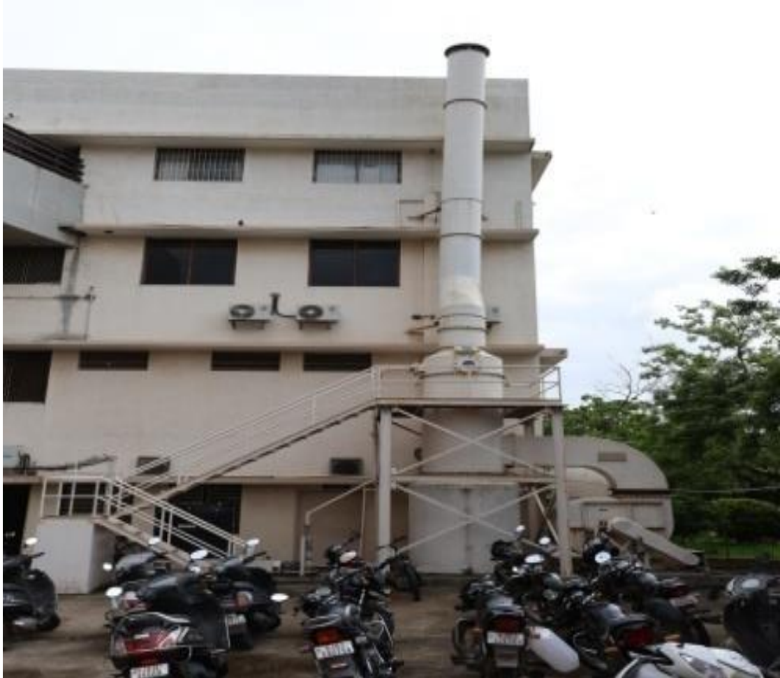
Wet Gas Scrubber
