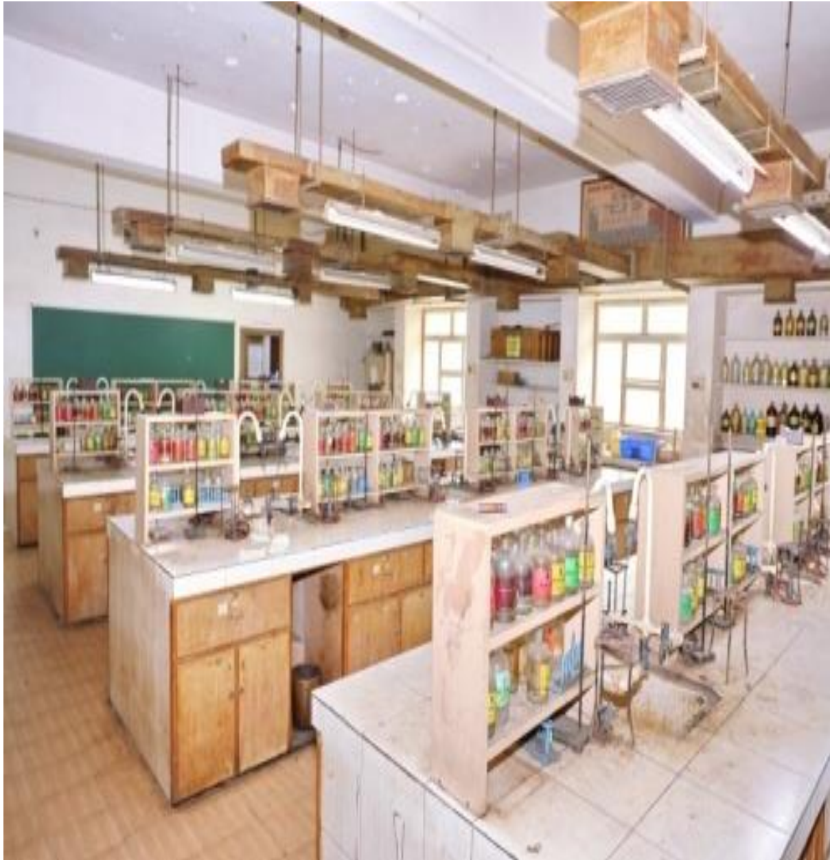
Acidic Fume Suction Panel
