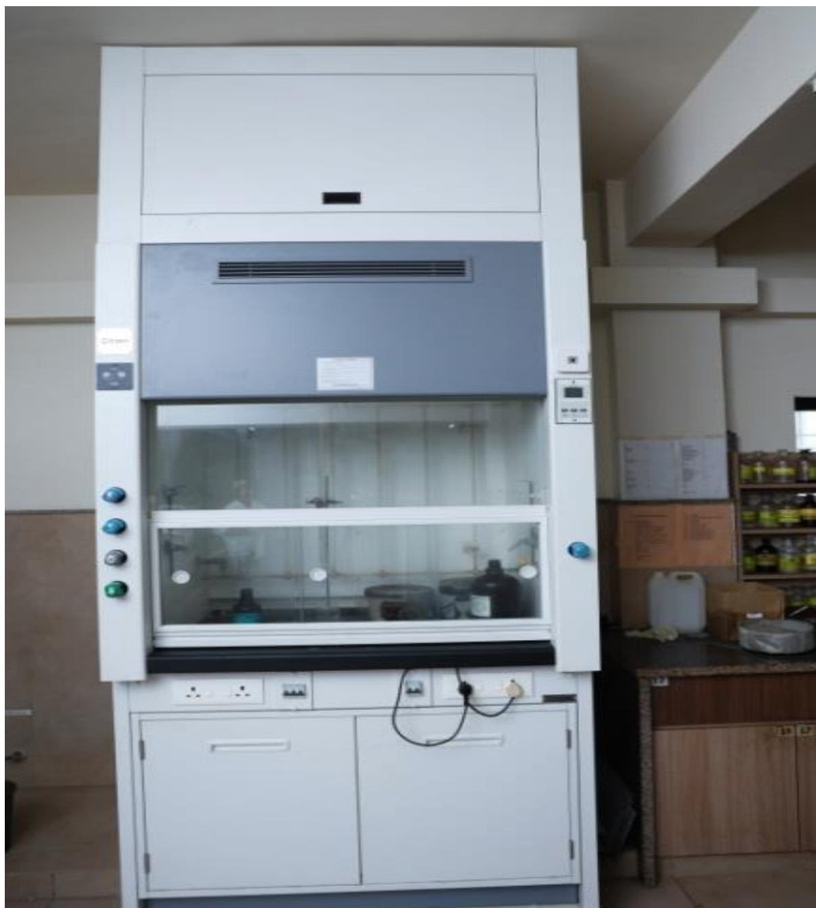
Fumehood at Chemistry Laboratory
