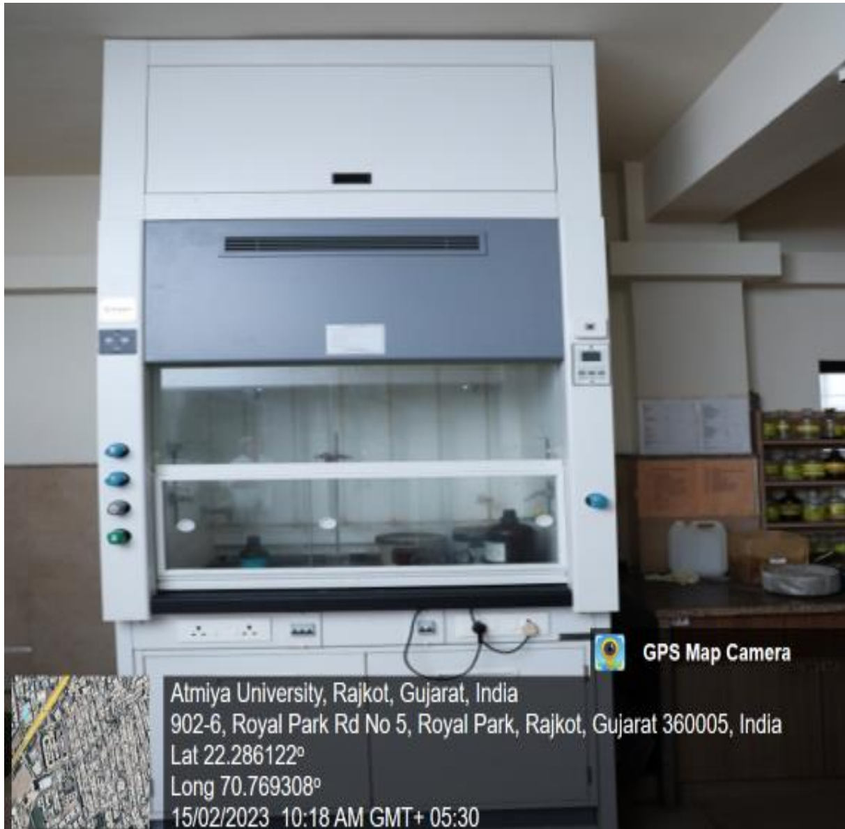
Fumehood at Chemistry Laboratory
