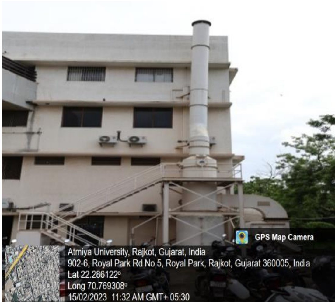
Wet Gas Scrubber
