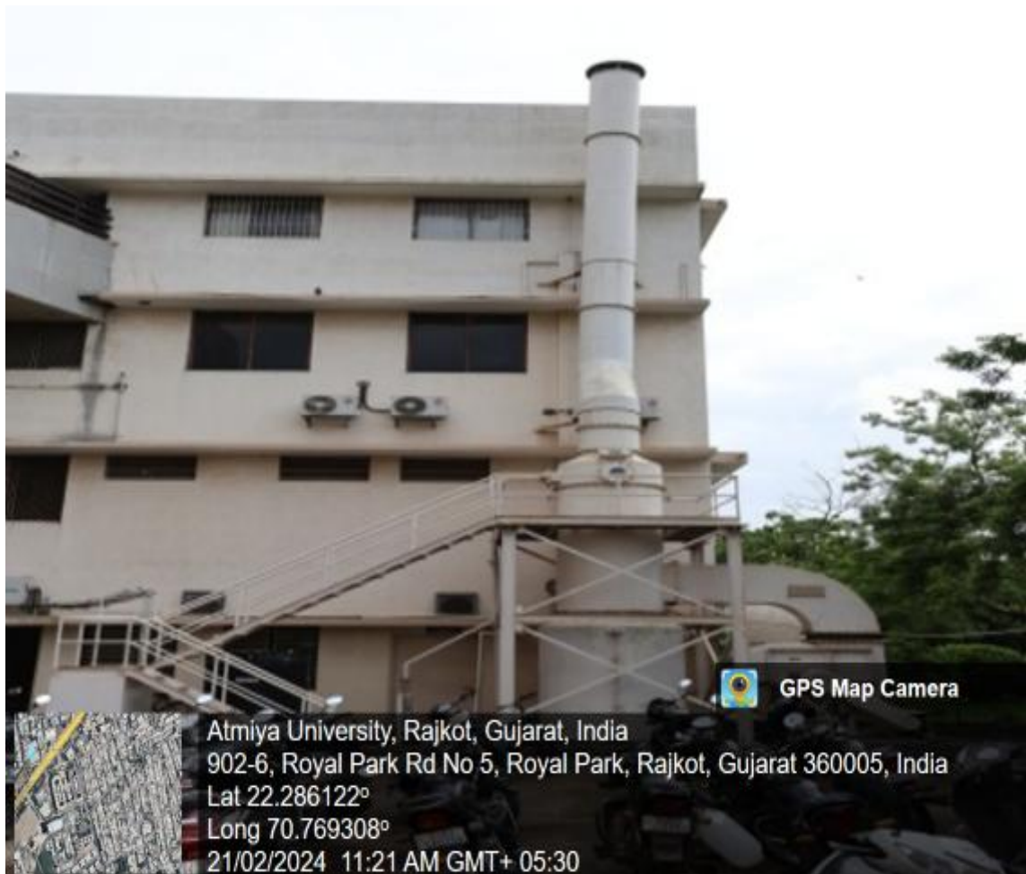
Wet Gas Scrubber
