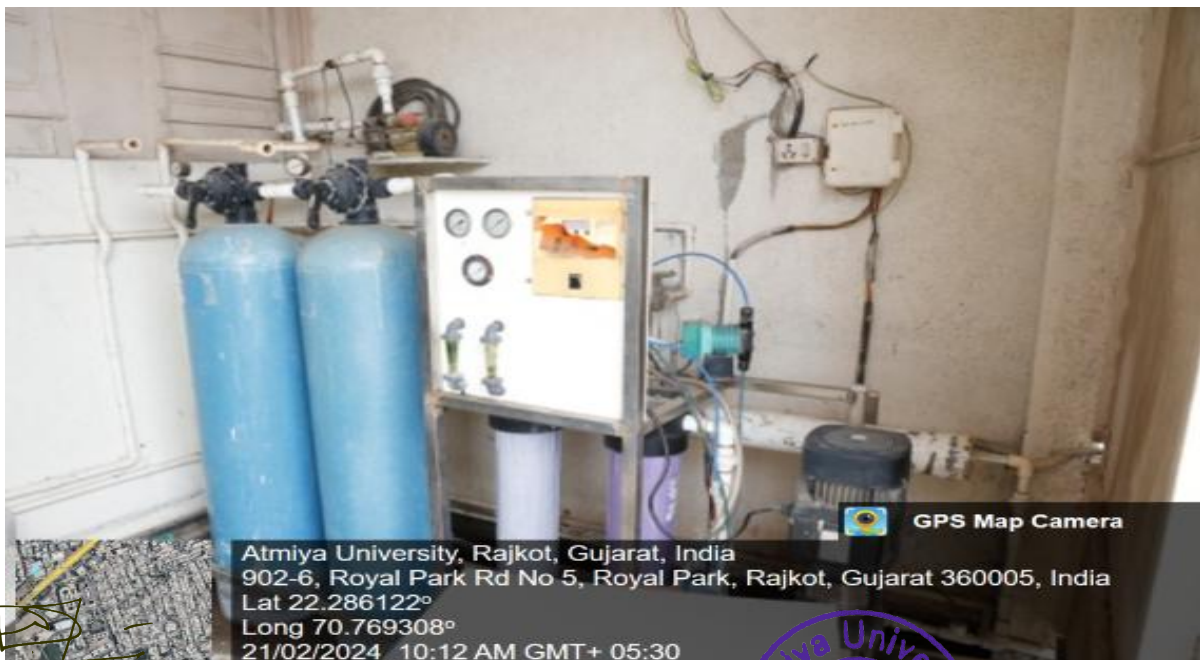
Reverse Osmosis Plant for Drinking Water
