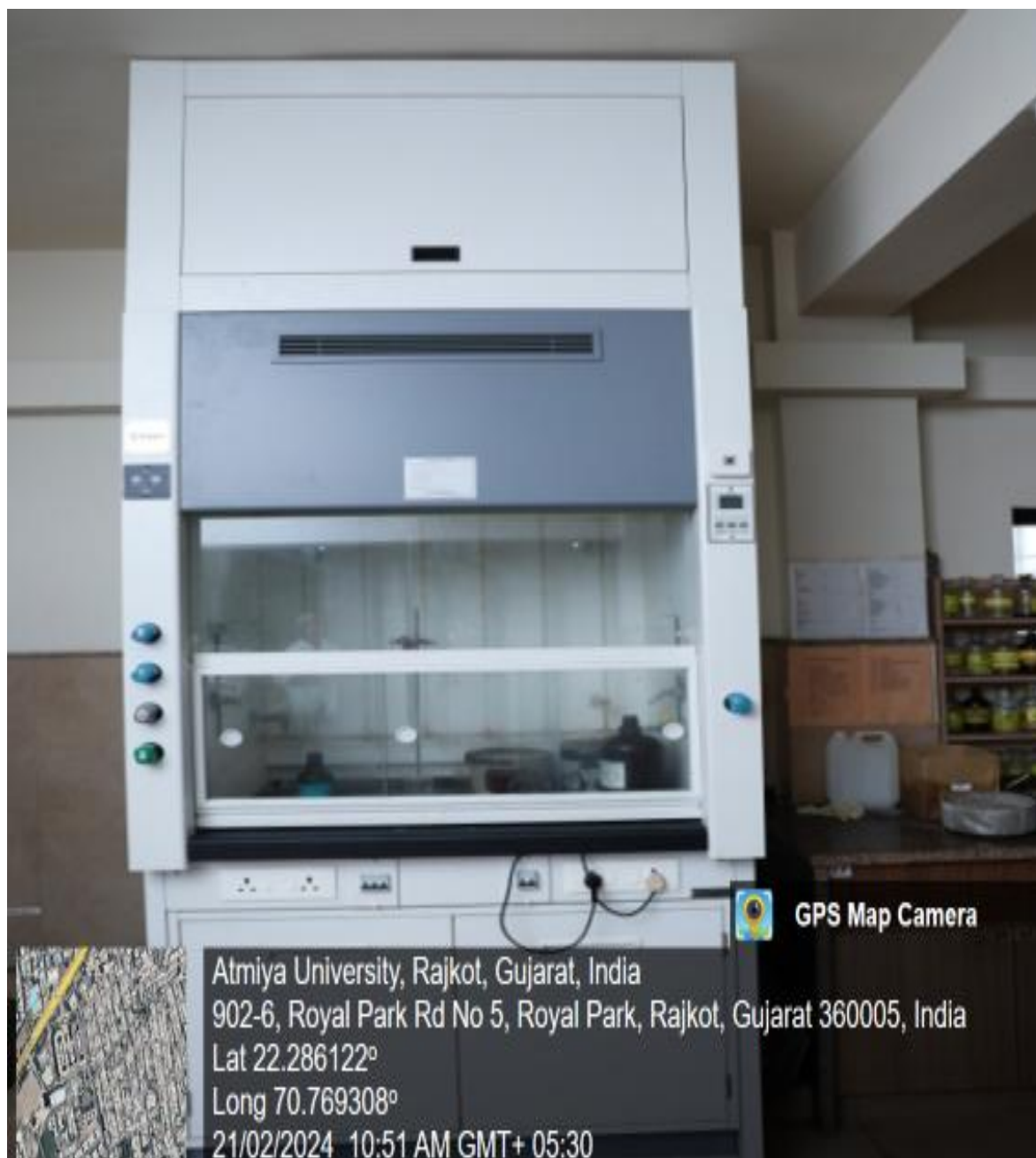
Fumehood at Chemistry Laboratory
