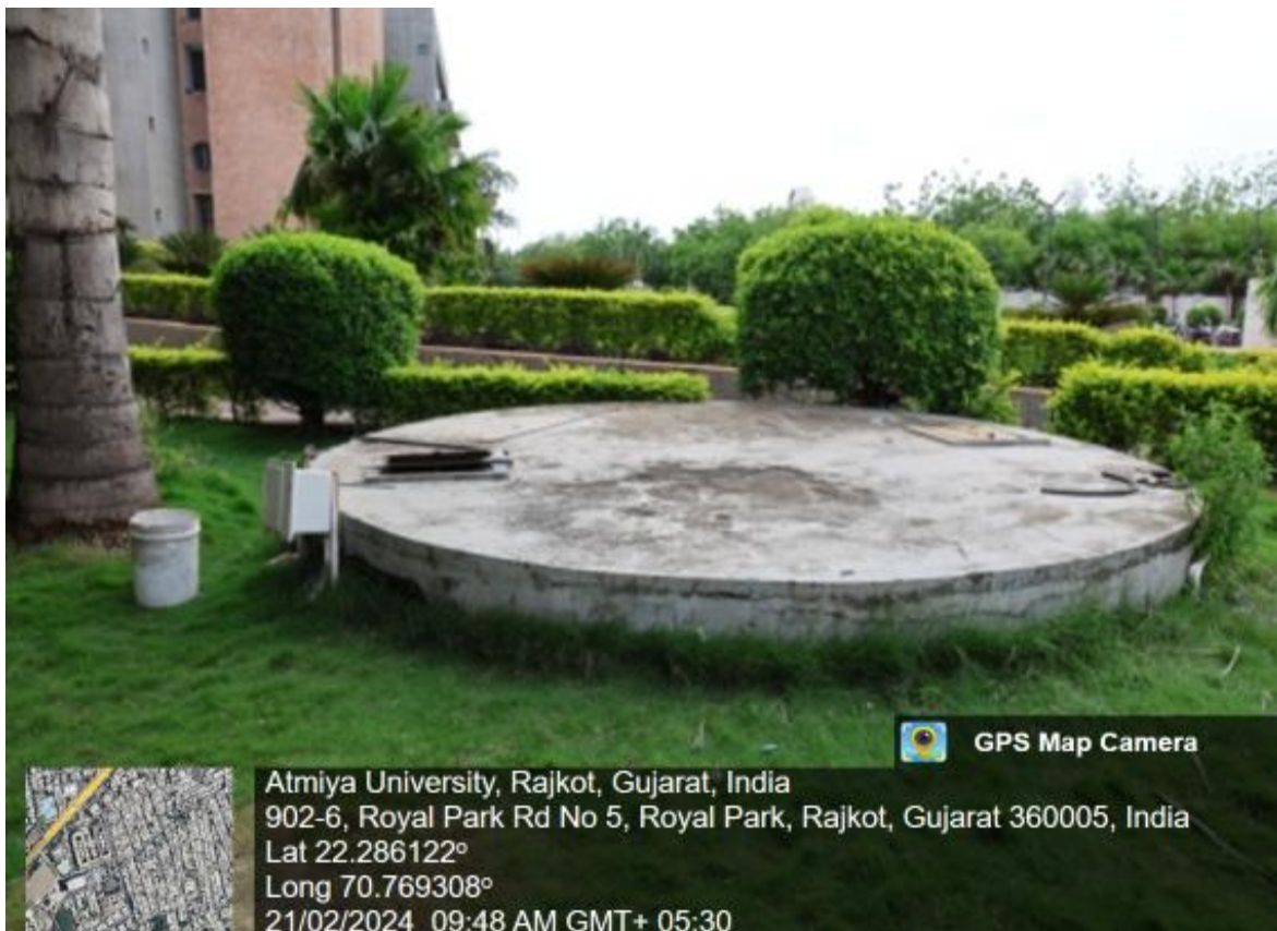
Rainwater Harvesting Tank
