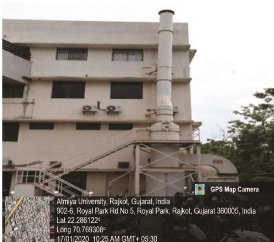
Wet Gas Scrubber
