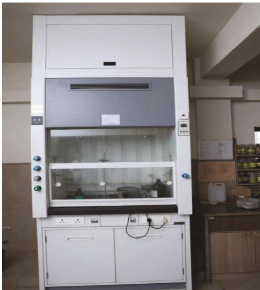
Fumehood at Chemistry Laboratory
