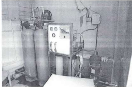
Reverse Osmosis Plant for Drinking Water
