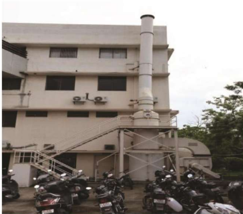
Wet Gas Scrubber
