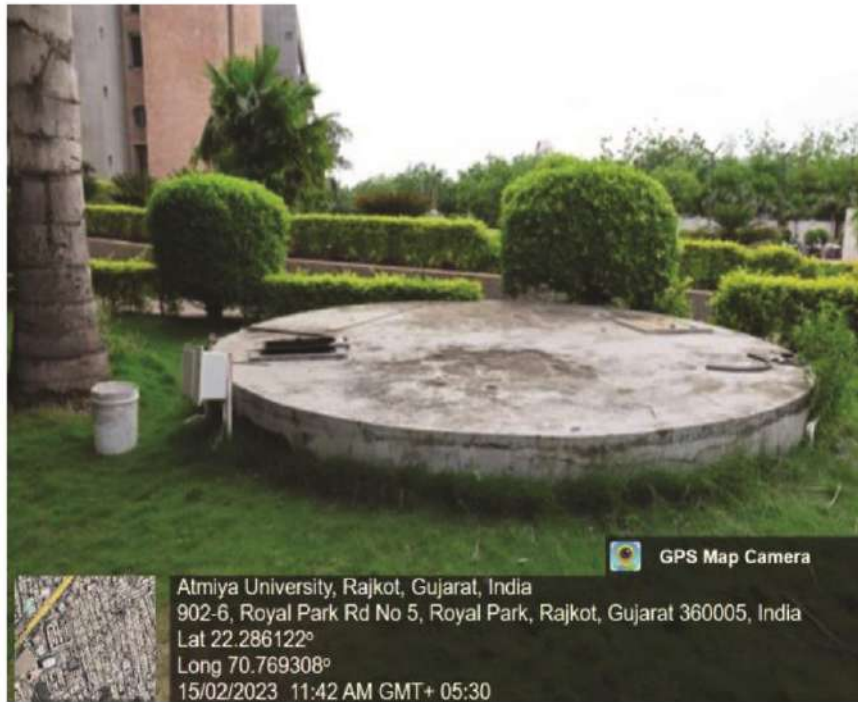
Rainwater Harvesting Tank
