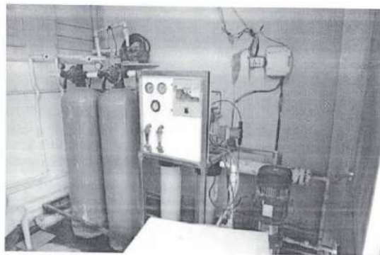
Reverse Osmosis Plant for Drinking Water
