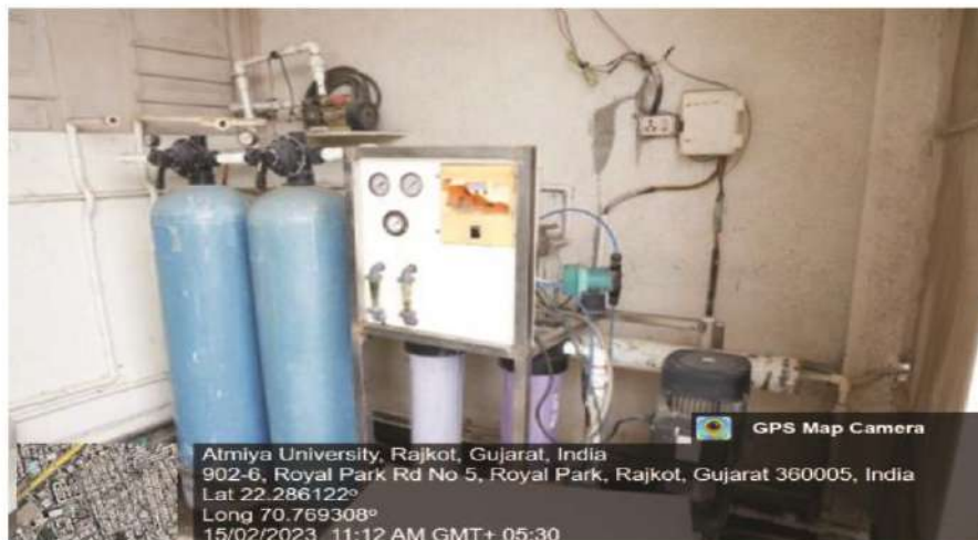
Reverse Osmosis Plant for Drinking Water
