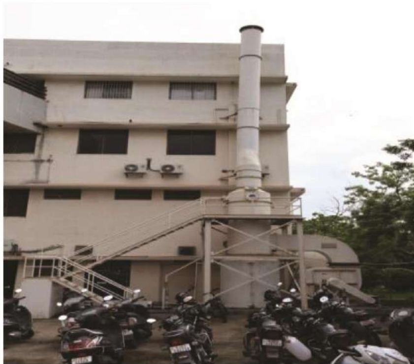
Wet Gas Scrubber
