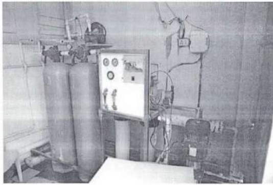
Reverse Osmosis Plant for Drinking Water
