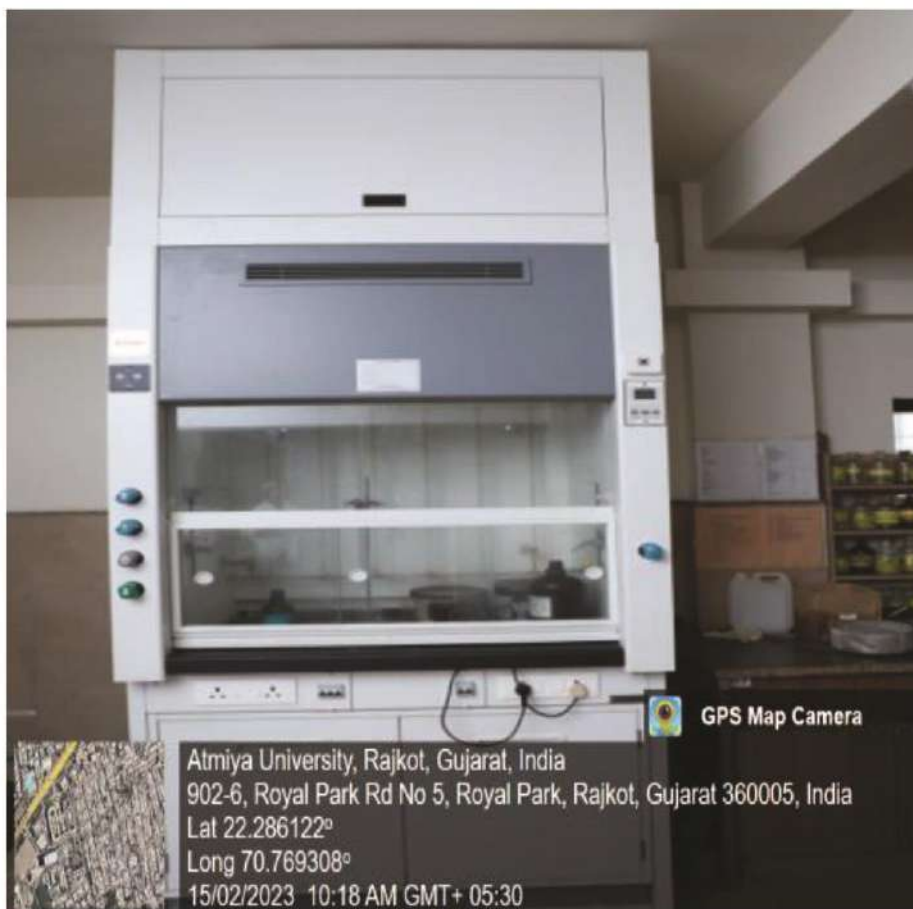
Fumehood at Chemistry Laboratory
