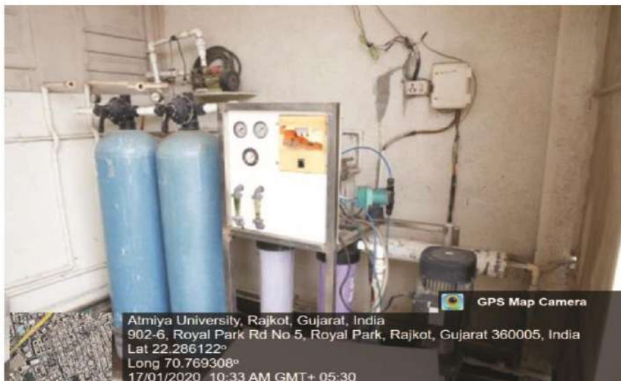
Reverse Osmosis Plant for Drinking Water
