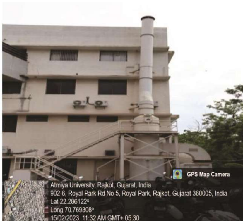
Wet Gas Scrubber
