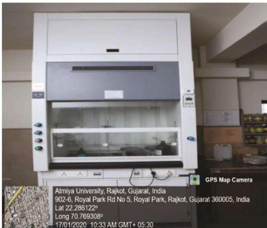
Fumehood at Chemistry Laboratory
