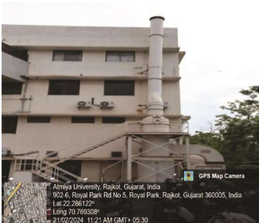
Wet Gas Scrubber
