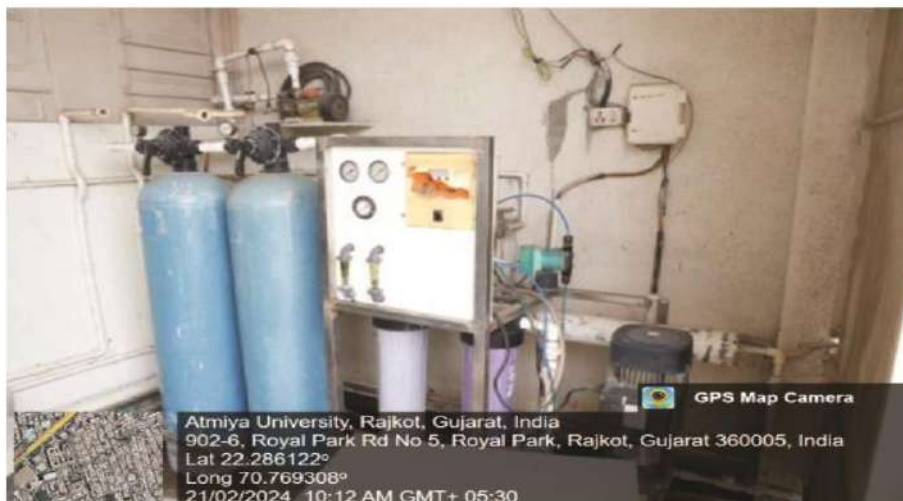
Reverse Osmosis Plant for Drinking Water
