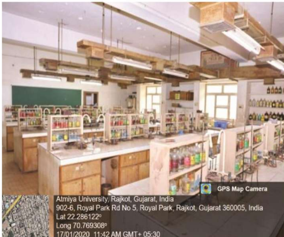
Acidic Fume Suction Panel
