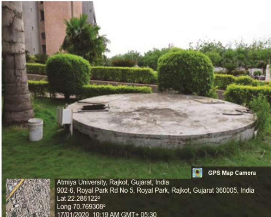
Rainwater Harvesting Tank
