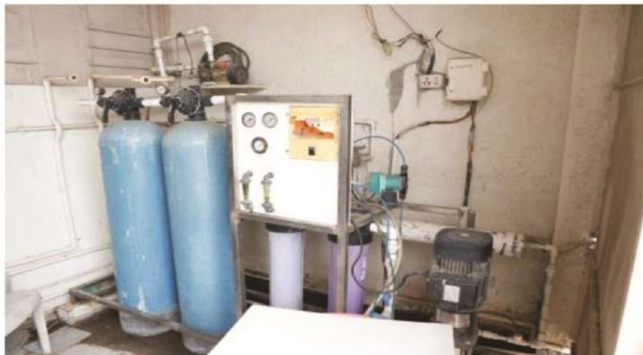
Reverse Osmosis Plant for Drinking Water
