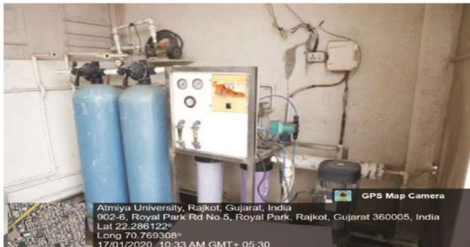
Reverse Osmosis Plant for Drinking Water
