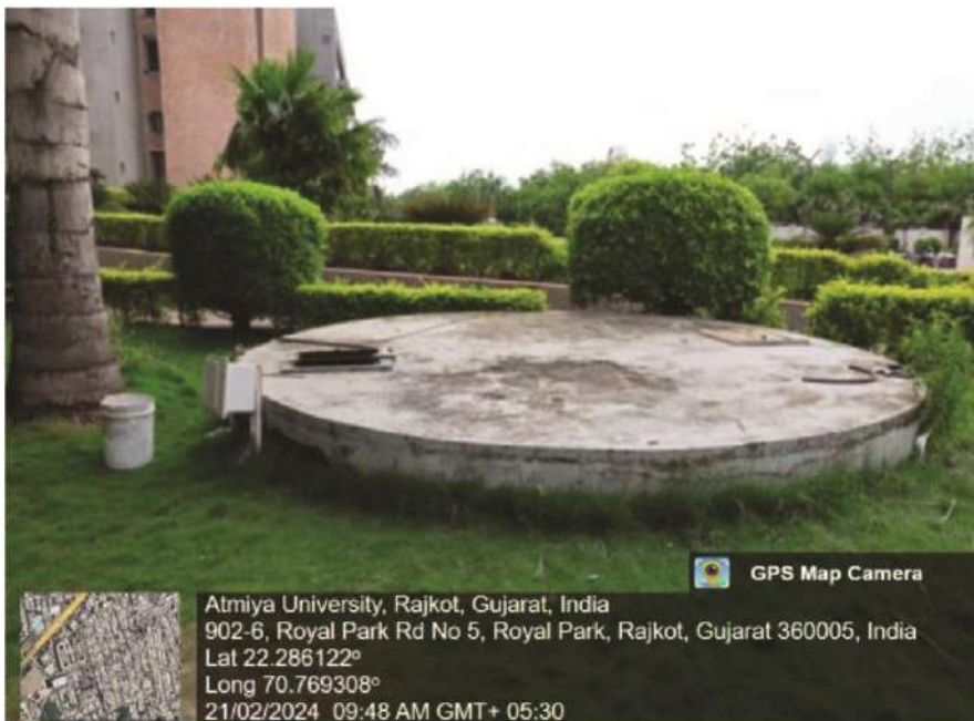
Rainwater Harvesting Tank
