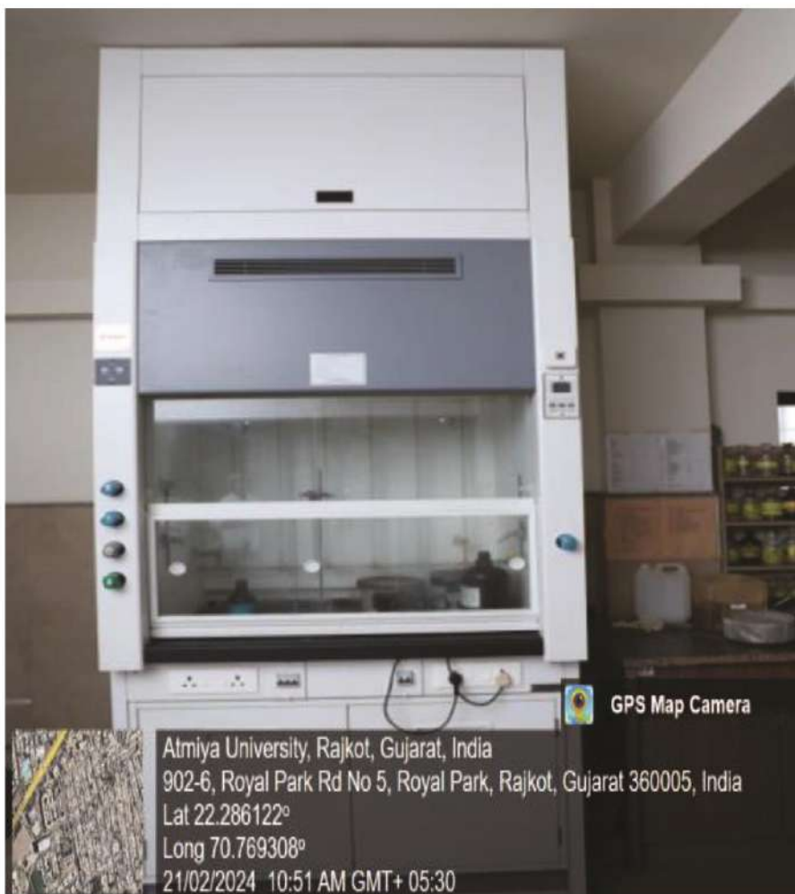
Fumehood at Chemistry Laboratory
