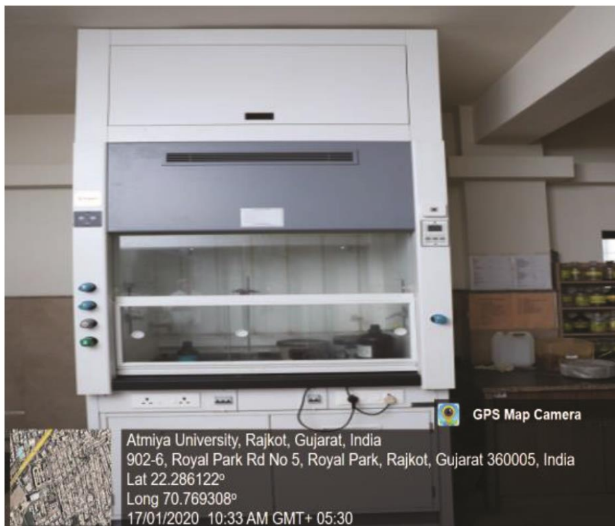
Fumehood at Chemistry Laboratory
