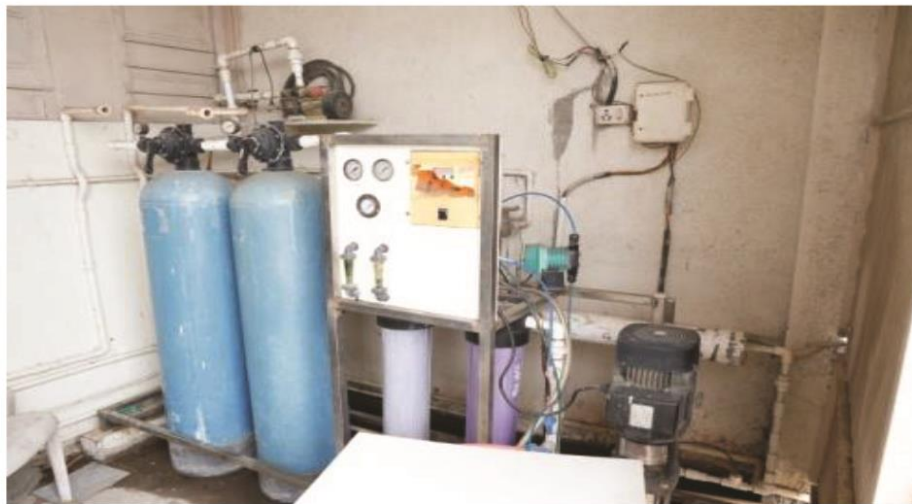
Reverse Osmosis Plant for Drinking Water
