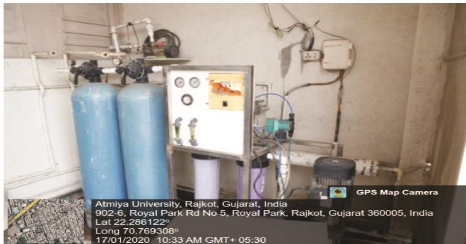
Reverse Osmosis Plant for Drinking Water
