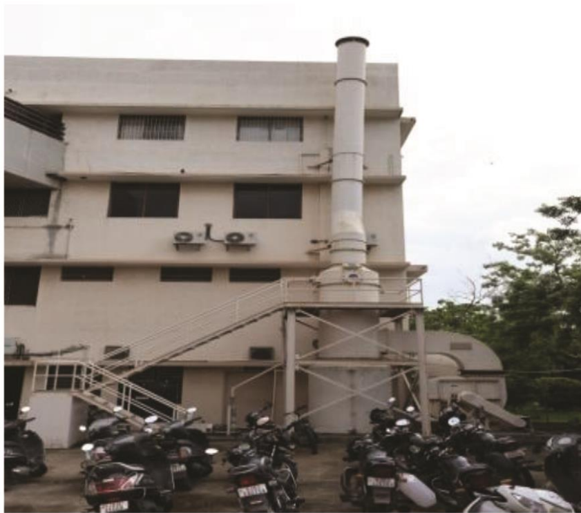
Wet Gas Scrubber
