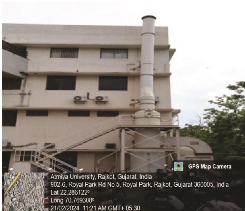
Wet Gas Scrubber
