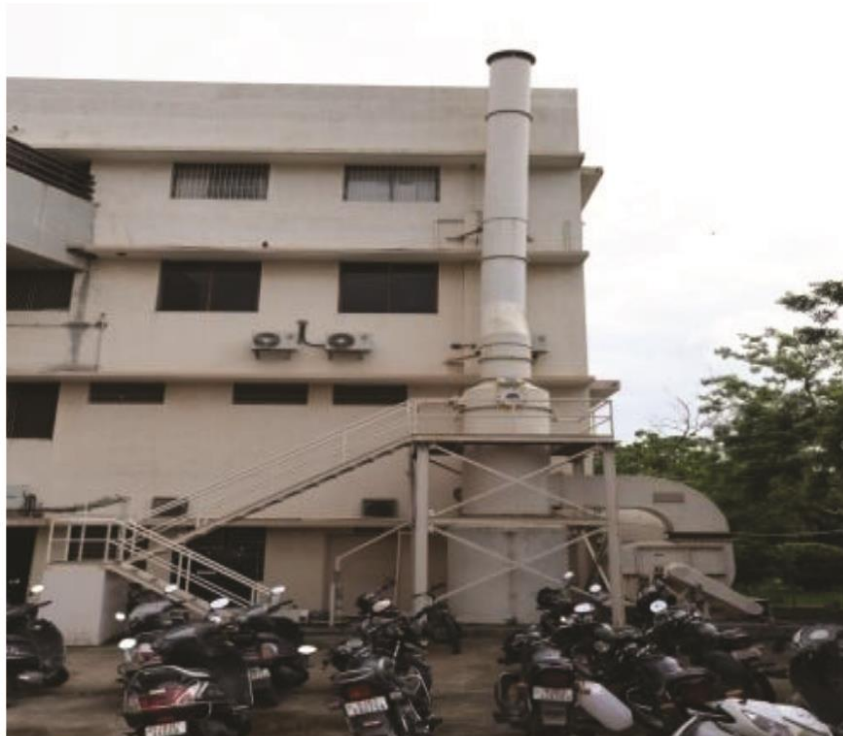
Wet Gas Scrubber
