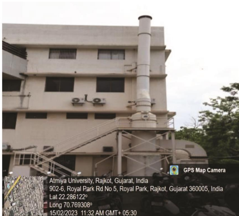
Wet Gas Scrubber
