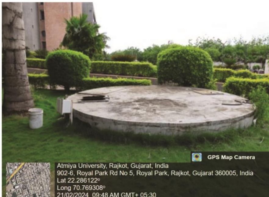
Rainwater Harvesting Tank
