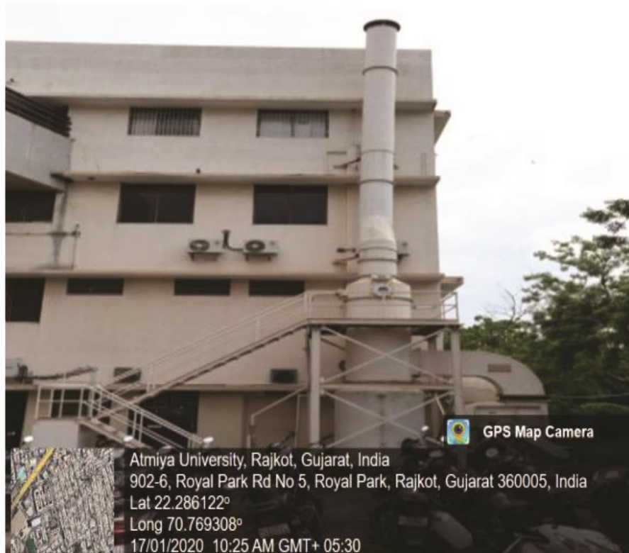
Wet Gas Scrubber
