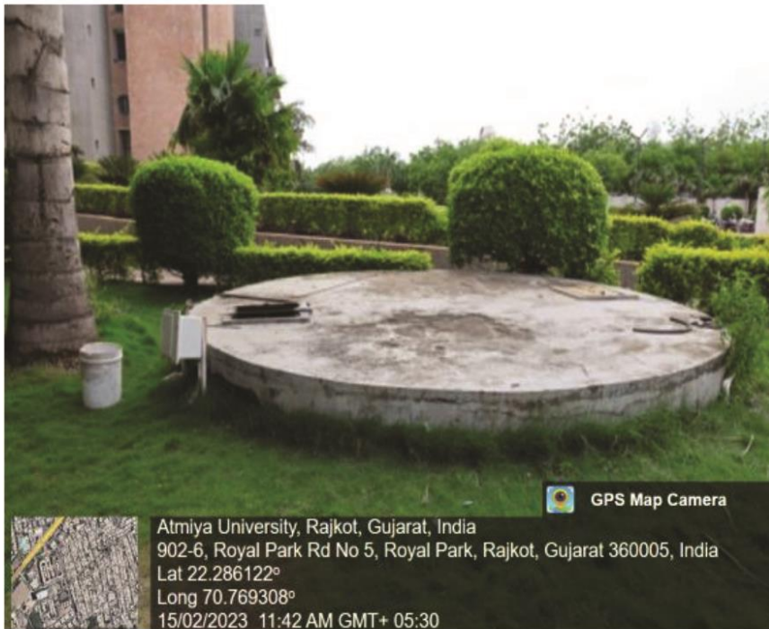
Rainwater Harvesting Tank
