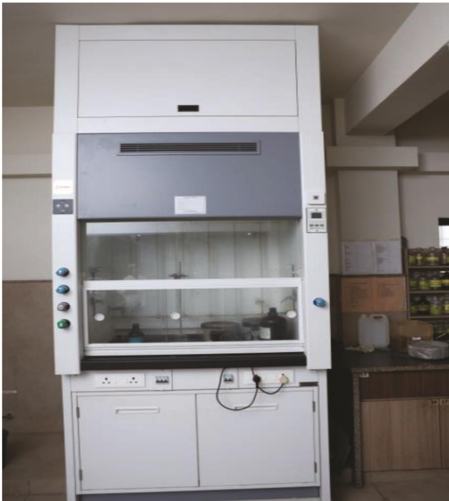
Fumehood at Chemistry Laboratory
