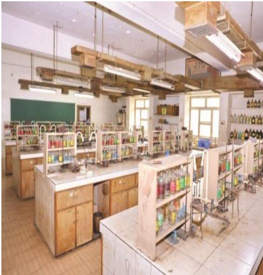
Acidic Fume Suction Panel
