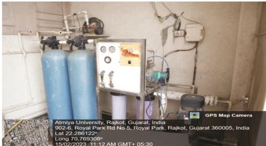
Reverse Osmosis Plant for Drinking Water
