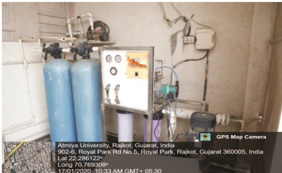
Reverse Osmosis Plant for Drinking Water
