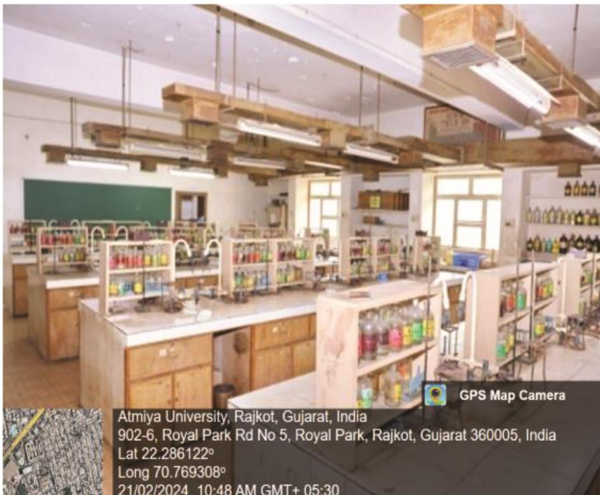
Acidic Fume Suction Panel
