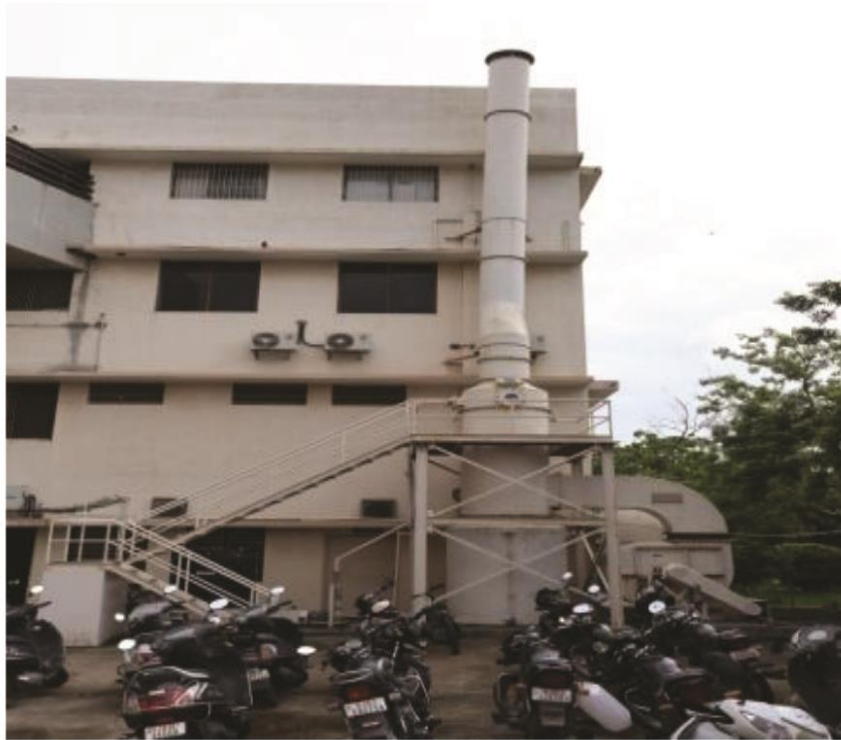
Wet Gas Scrubber
