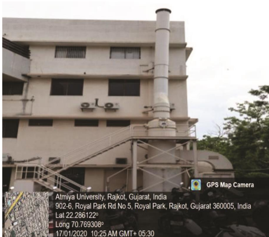
Wet Gas Scrubber
