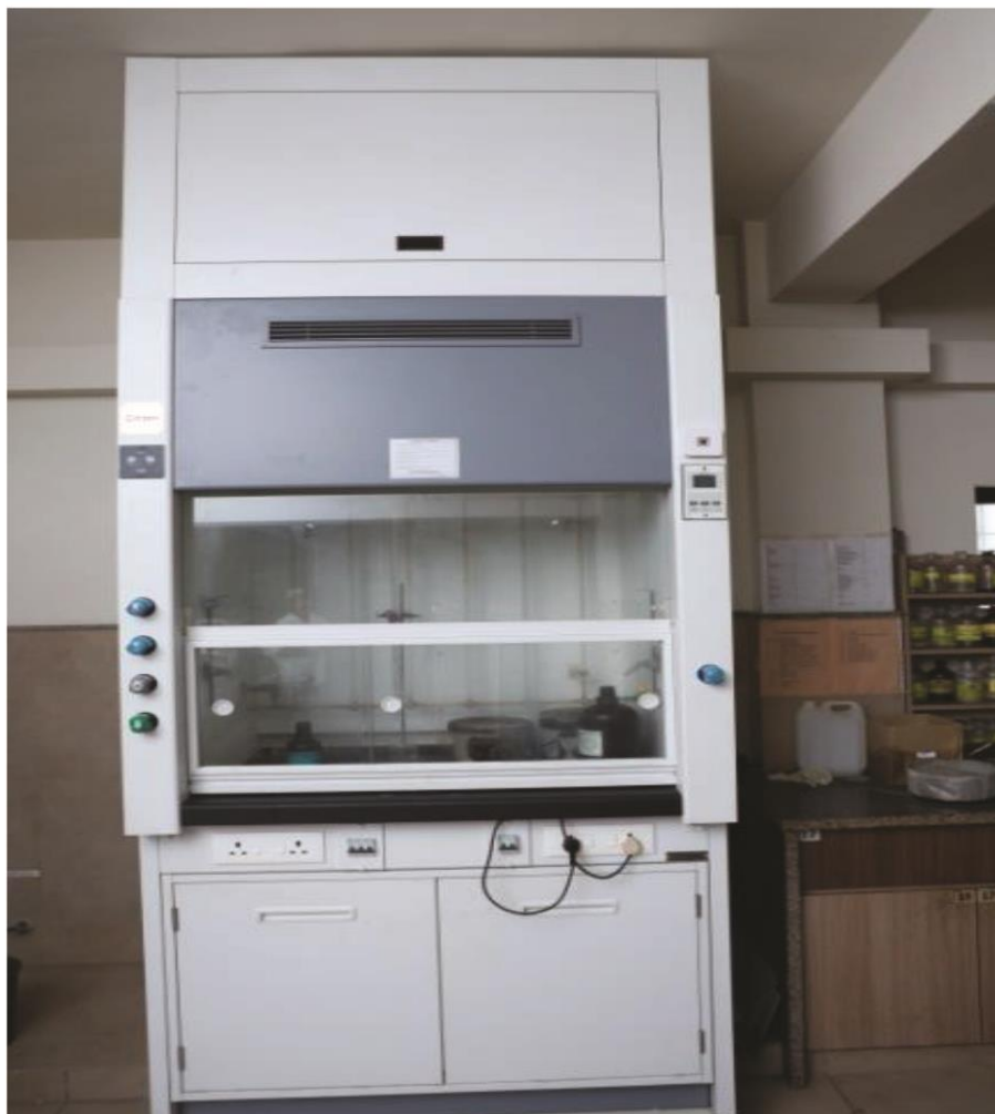
Fumehood at Chemistry Laboratory
