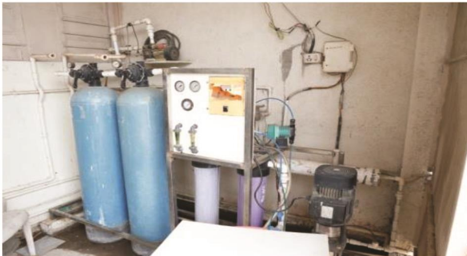
Reverse Osmosis Plant for Drinking Water
