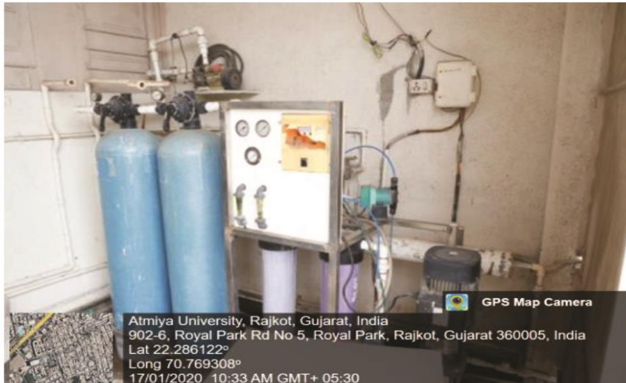
Reverse Osmosis Plant for Drinking Water
