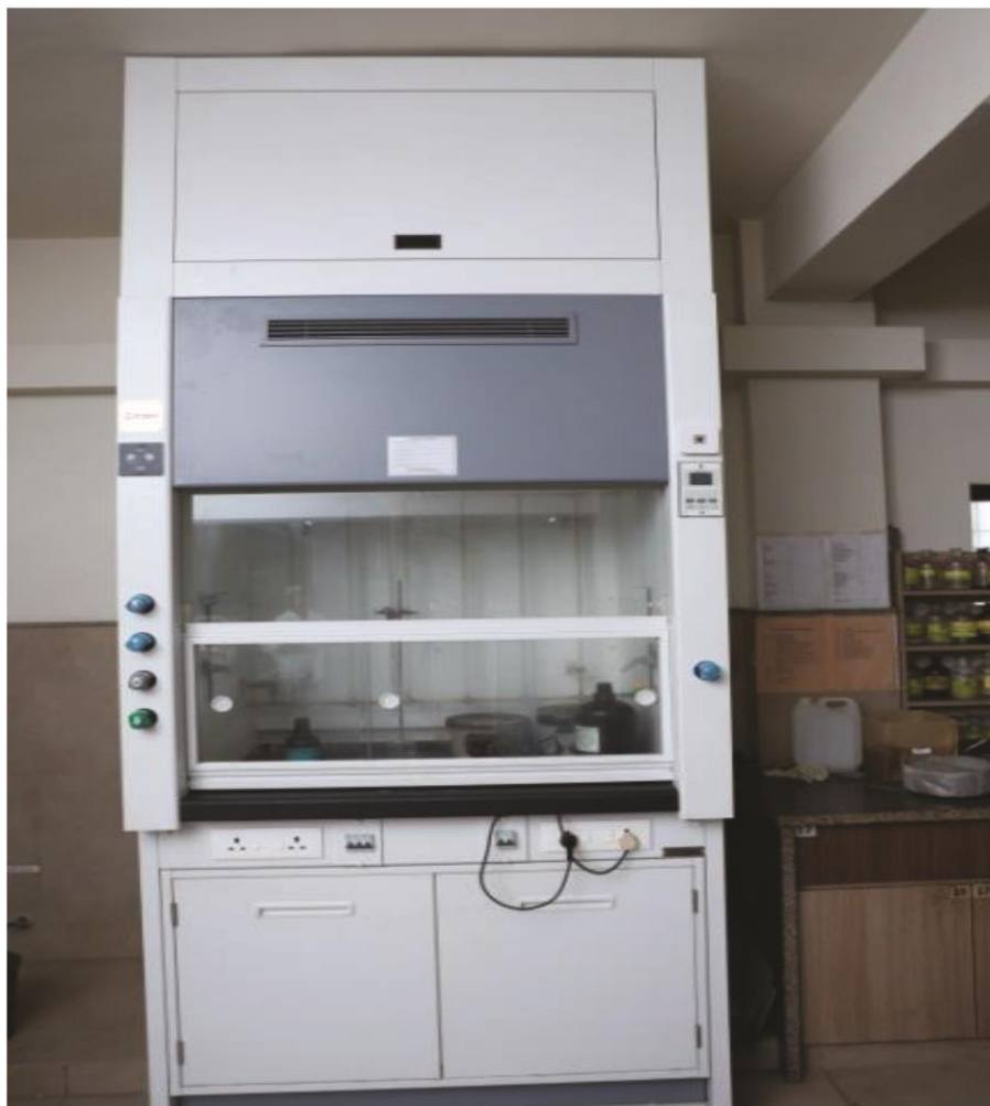
Fumehood at Chemistry Laboratory
