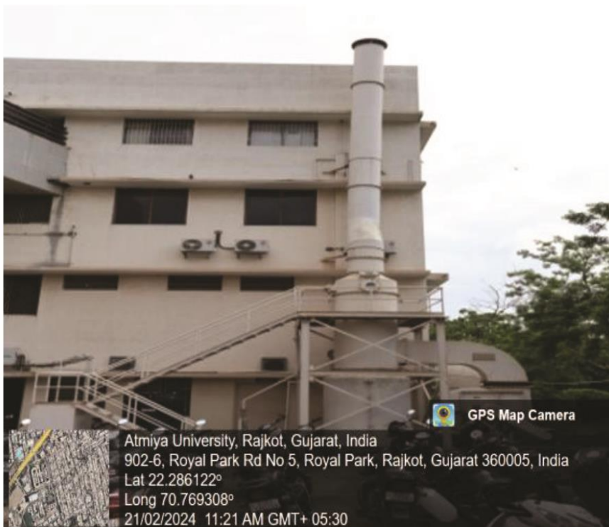
Wet Gas Scrubber
