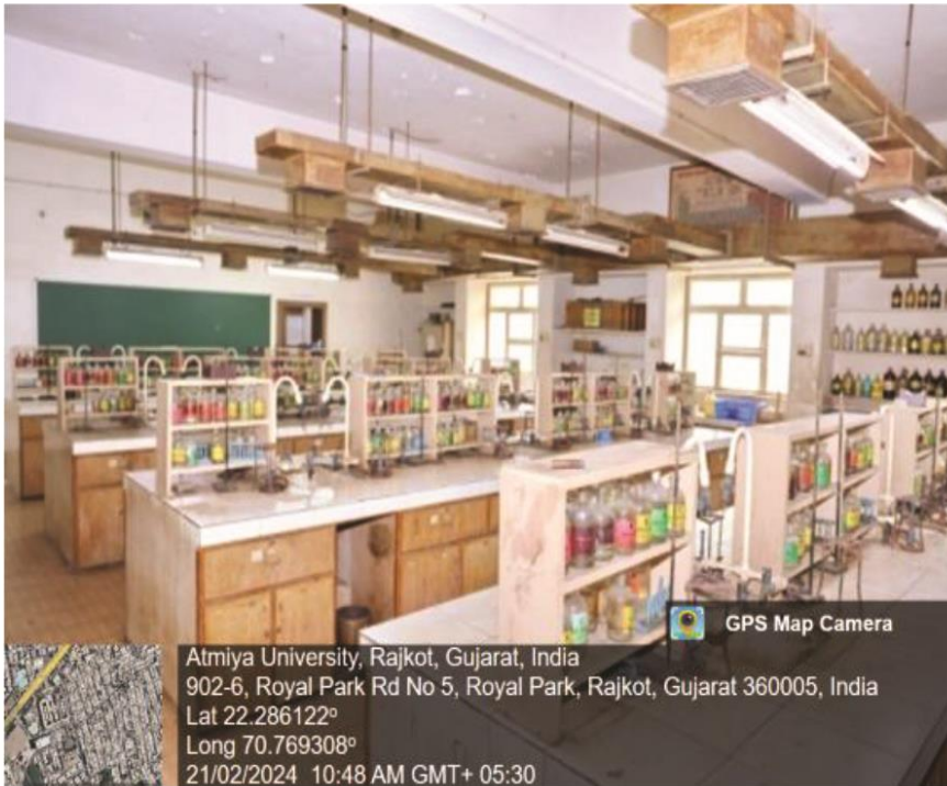
Acidic Fume Suction Panel
