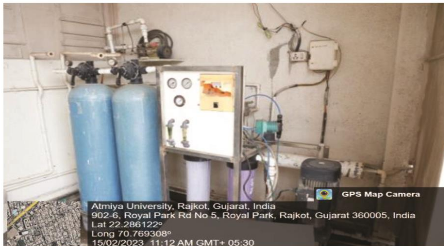
Reverse Osmosis Plant for Drinking Water
