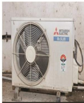
Power Efficient Equipment – 5 Star Rated Appliances/ Equipment
