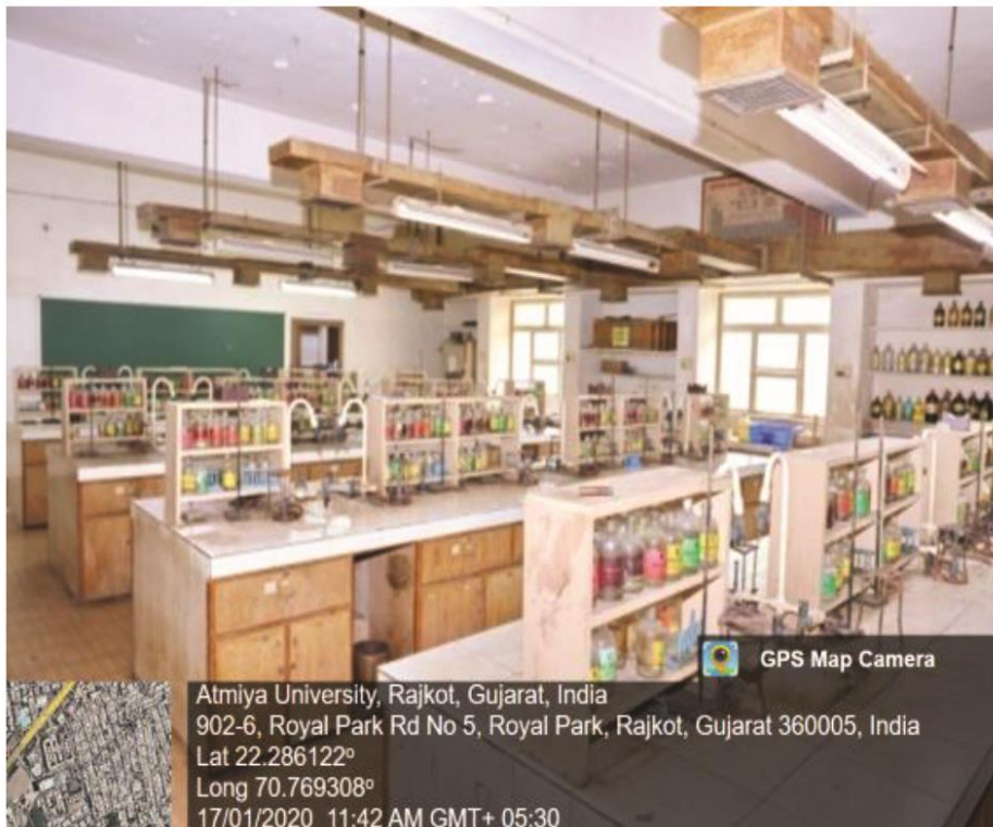
Acidic Fume Suction Panel
