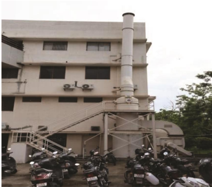
Wet Gas Scrubber
