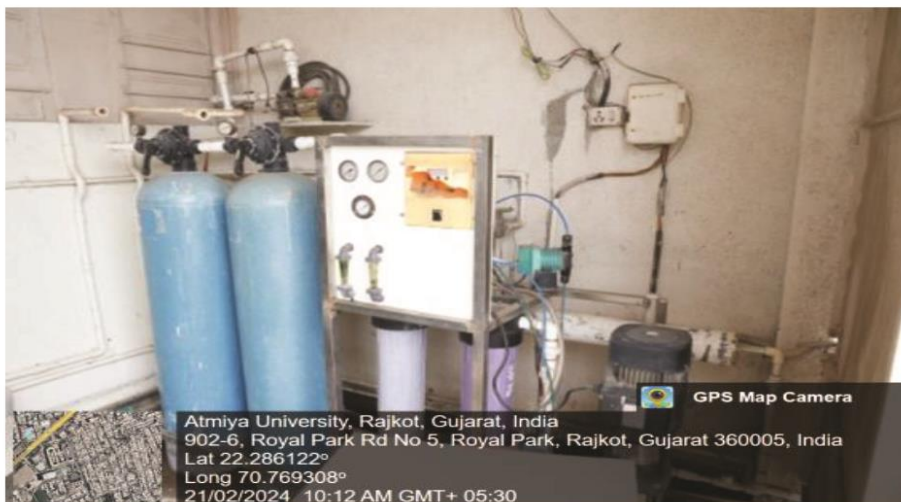
Reverse Osmosis Plant for Drinking Water Rainwater Harvesting
