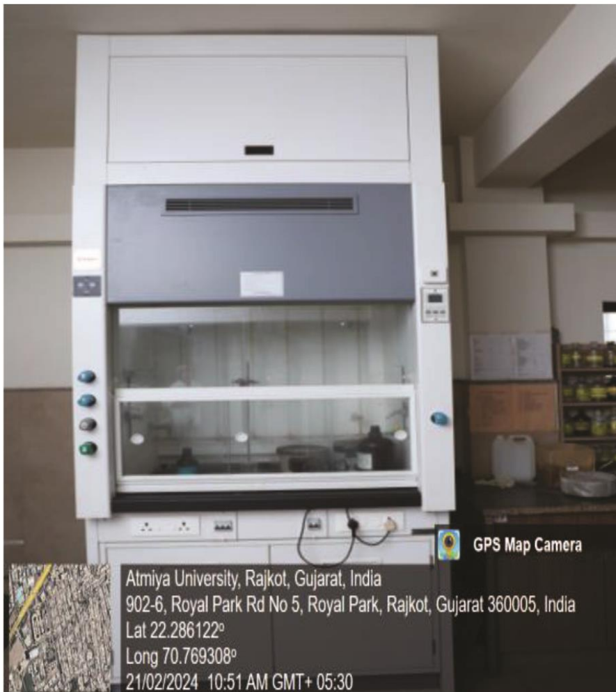
Fumehood at Chemistry Laboratory
