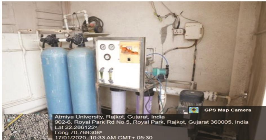
Reverse Osmosis Plant for Drinking Water
