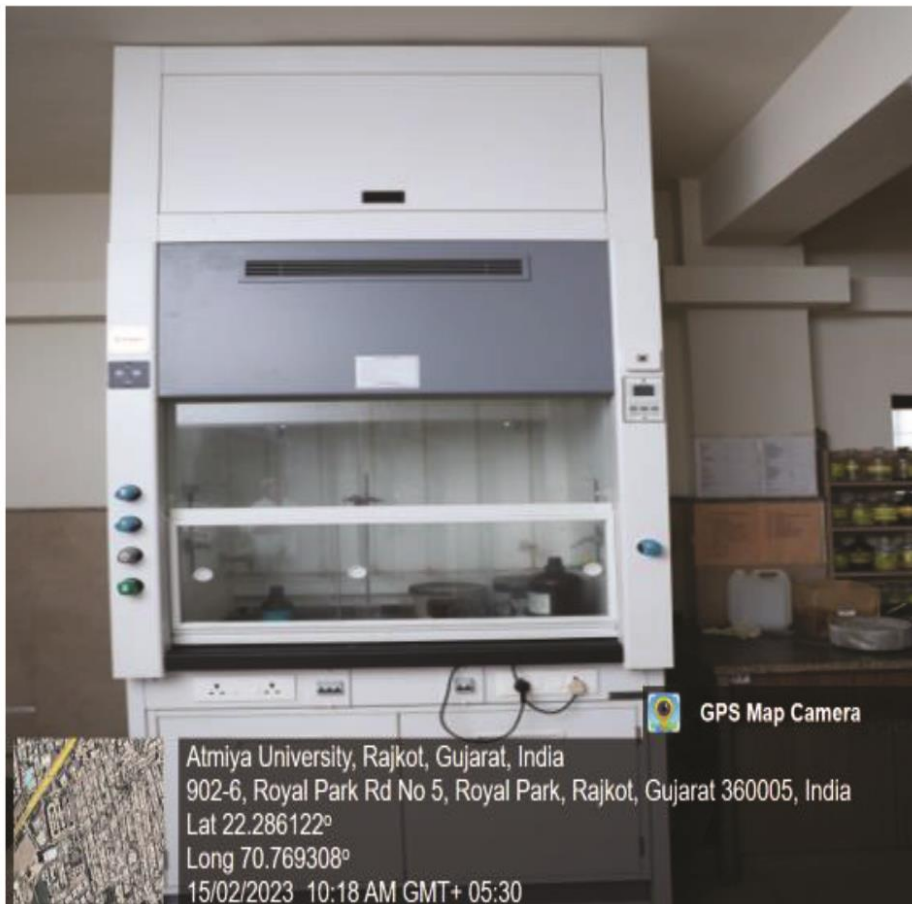
Fumehood at Chemistry Laboratory
