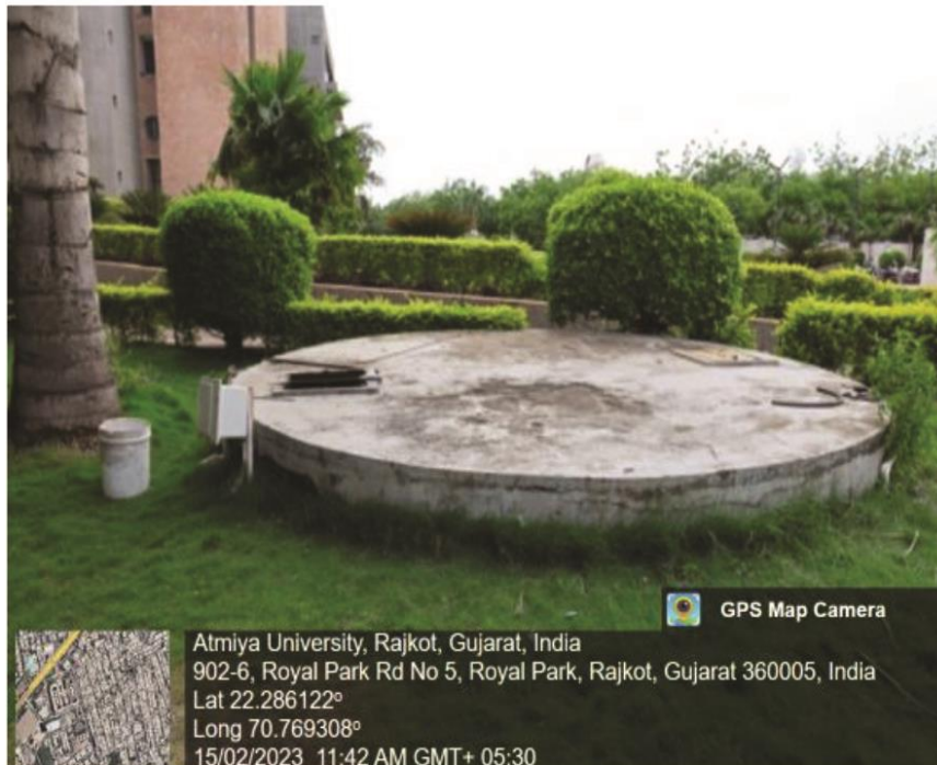
Rainwater Harvesting Tank
