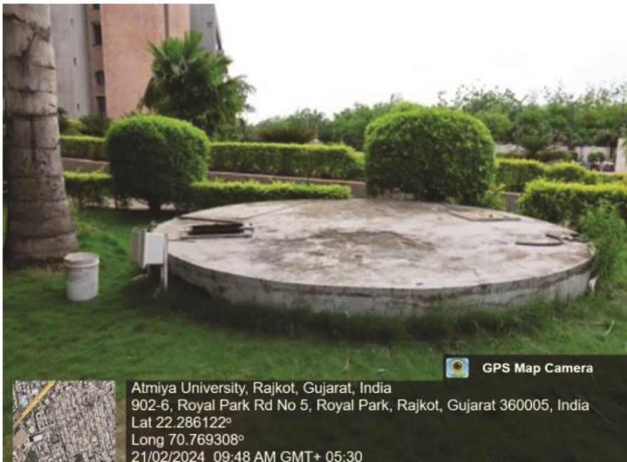
Rainwater Harvesting Tank
