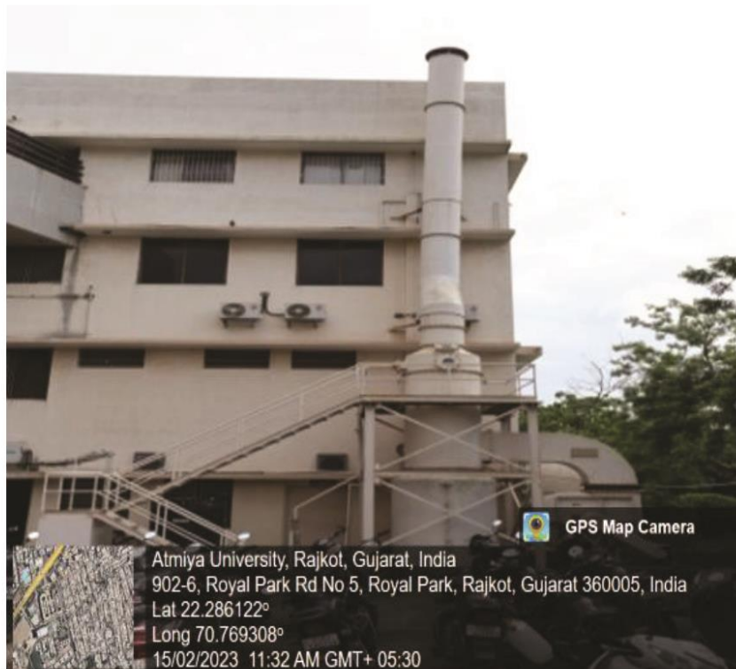
Wet Gas Scrubber
