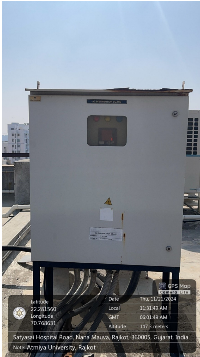
AC Distribution Board
