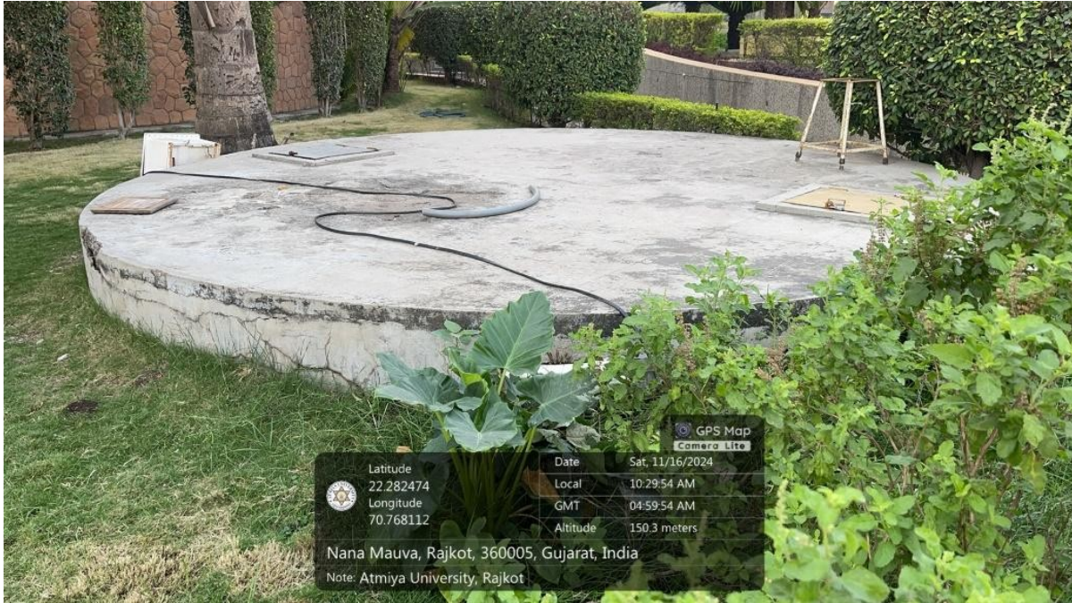
RO water tank and distribution system
